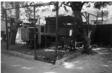
Fig. B26 : Outdoor substations without enclosures
